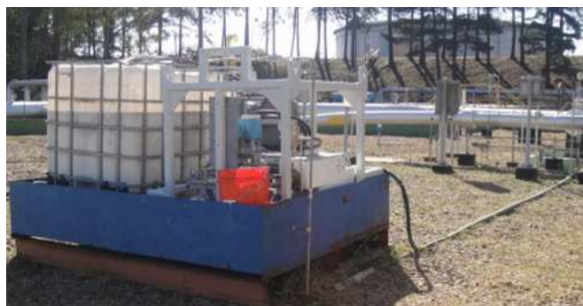
Figure 4 – Example of the Injection Skid Installed in the Field
